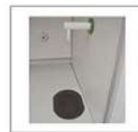
Water Tap & Water Sink
